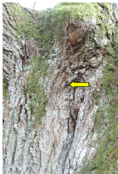
Figure 12. A drain that drains water from the inside of the tree trunk (photo by W. Durlak)
