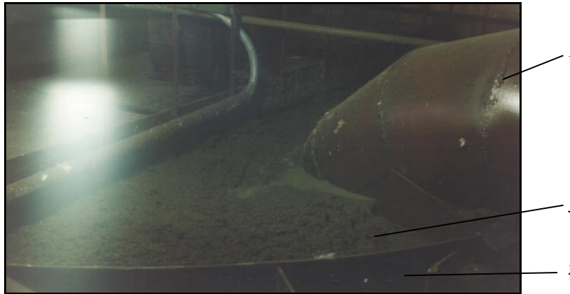
Phot. 3. Sludge from sludge separation device: 1 – sludge duct, 2 – the bunker-dehydrator; 3 – sludge (aut. V.I. Piskun)
